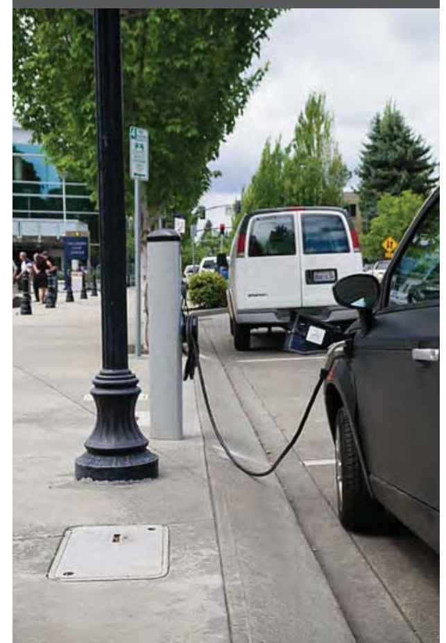
Figure 8-E Curbside Electric Vehicle Charging
