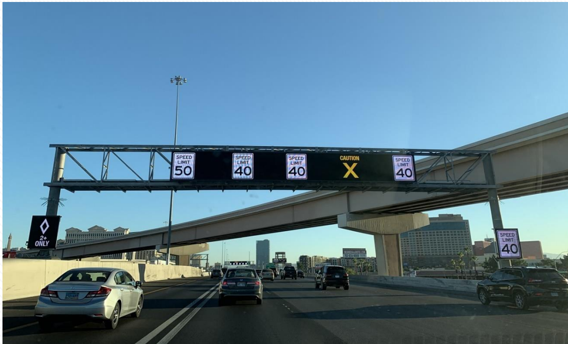
Figure 120: Active Traffic Management Sign installed in Southern Nevada
