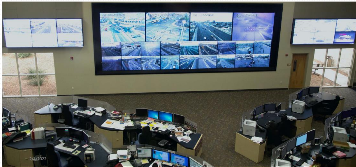
Figure 20: Picture of FAST Control Center
